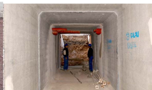
GALERIES SUBTERRANIES REGISTRABLES
